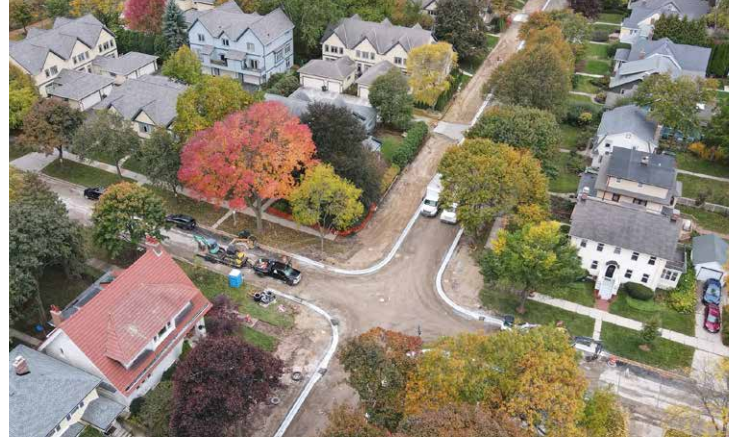
The intersection of North Prospect Avenue and East Stratford Court is the heart of an extensive construction zone that is part of the Village's largest-ever infrastructure project.
