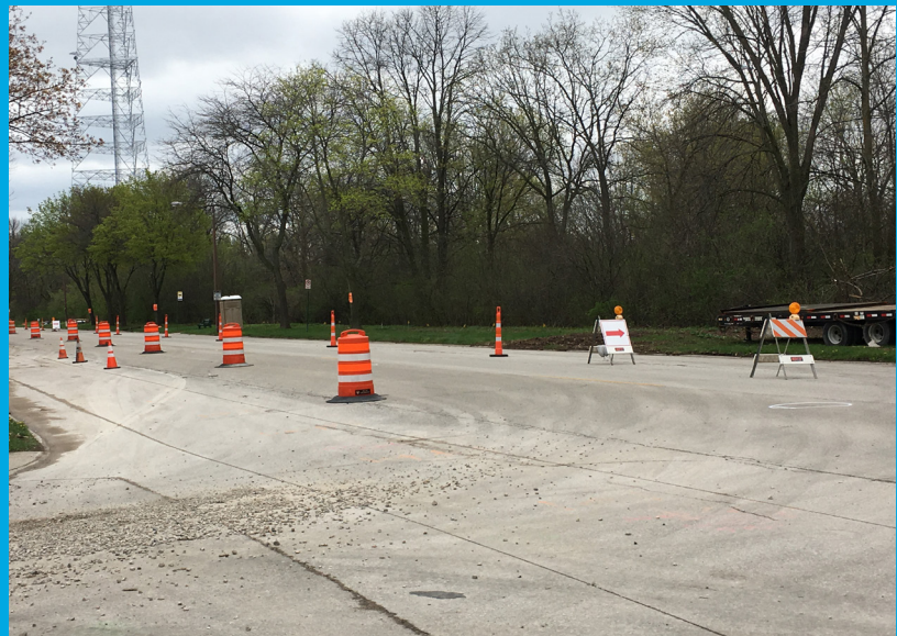
↑ Traffic between E. Olive St. and N. Marlborough Dr. has been moved to the existing southbound lane.
