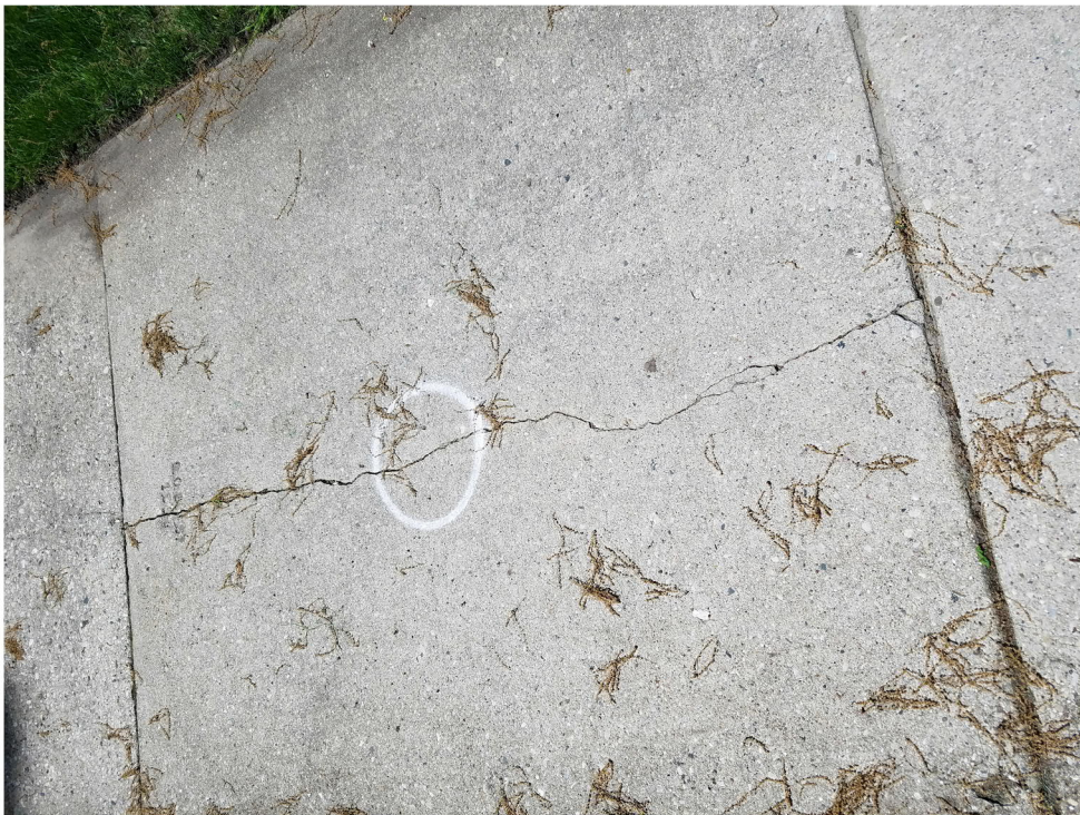
Criteria 3 - 1/4-inch Crack in the Slab
