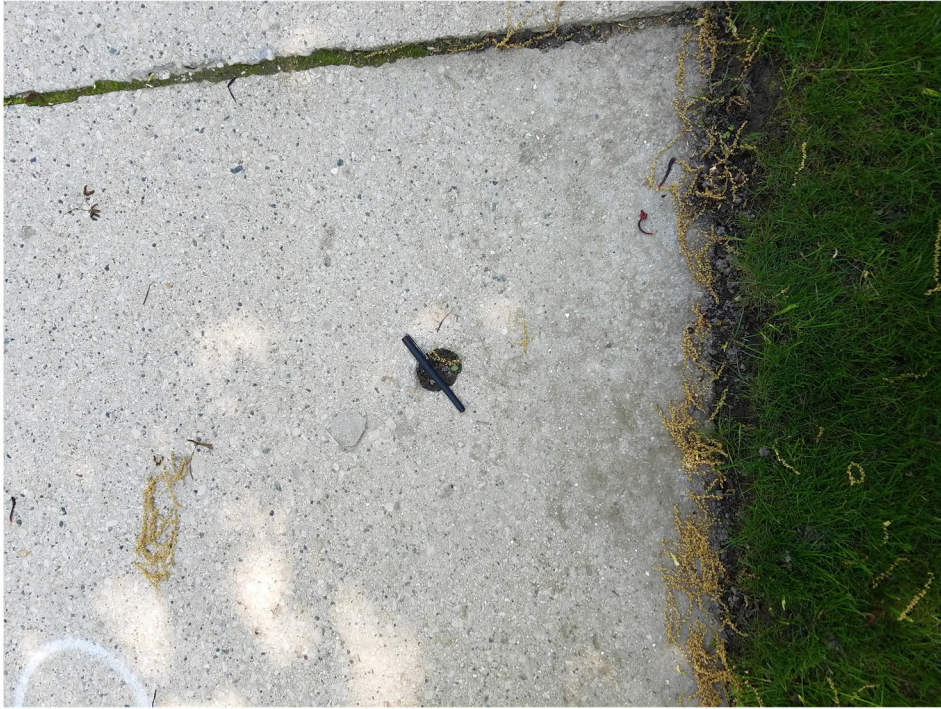
Criteria 2 - Example Mudjacking Hole that is not Sealed.
