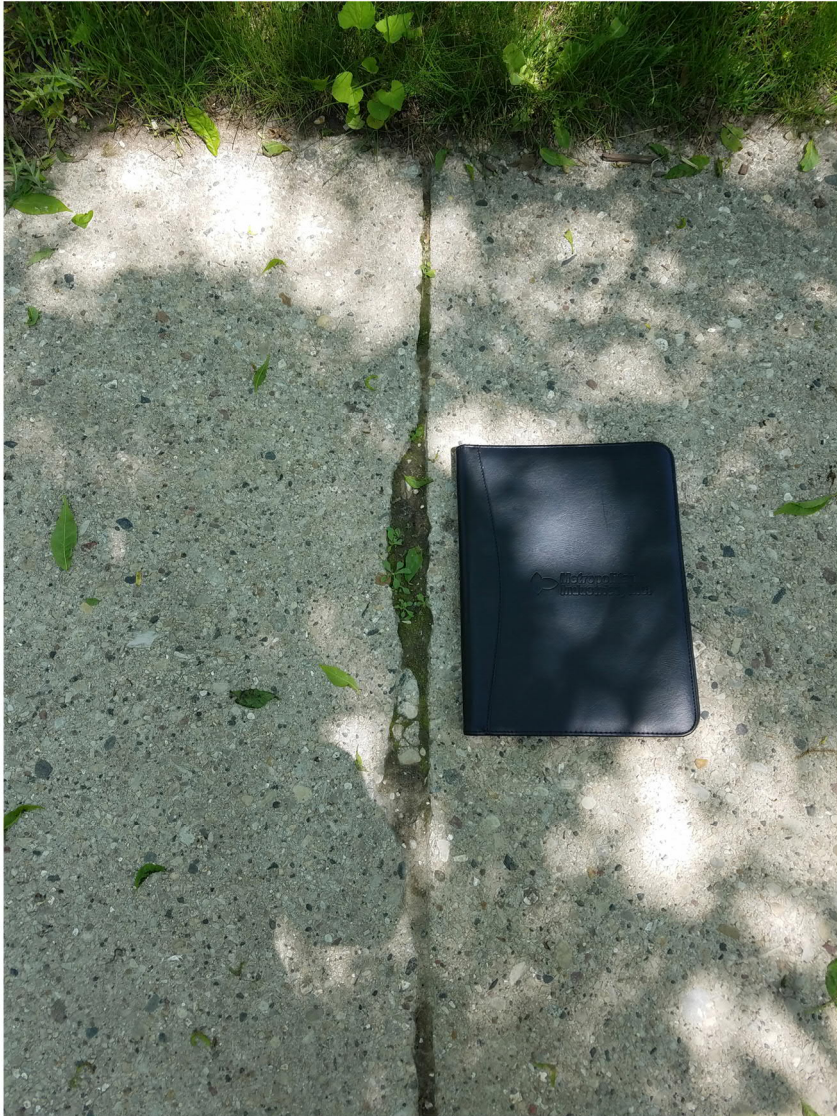
Criteria 1 - Defect at Control Joint Approximately 9-inches by 3-inches
