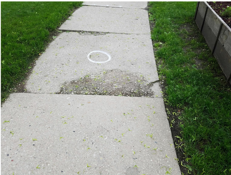
Criteria 5 - Crumbing Surface
