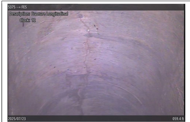
Figure 15 Grade 3 FL in Pipe Segment 5375-FES
