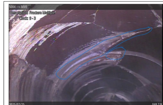
Figure 14 Grade 4 FM and Misalignment in Pipe Segment 5004-5005
