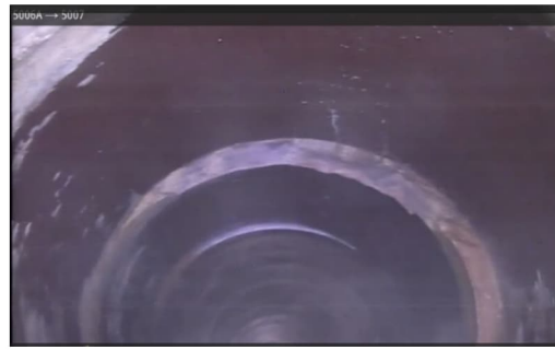
Figure 3 Pipe Misalignment in Segment 5006A-5007
