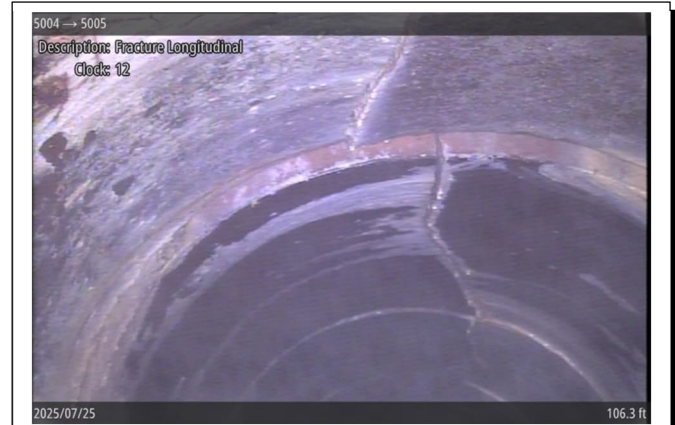
Figure 18 Grade 4 FM and Misalignment in Pipe Segment 5004-5005
