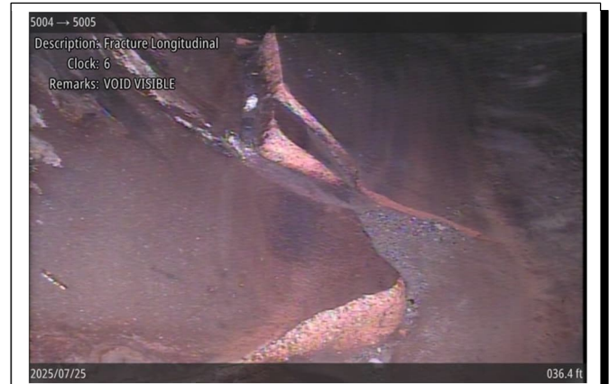
Figure 16 Grade 3 FL and Protrusion in Pipe Segment 5004-5005
