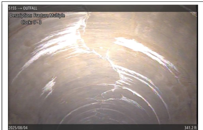
Figure 11 Grade 4 FM in Pipe Segment 5155-OUTFALL
