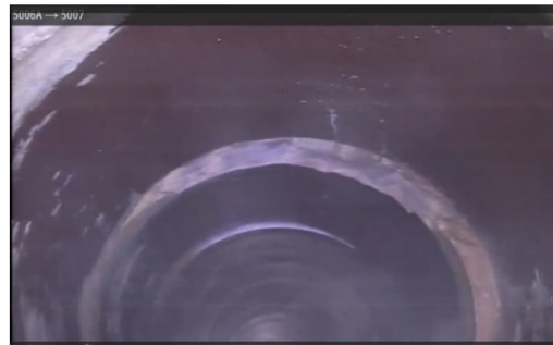
Figure 3 Pipe Misalignment in Segment 5006A-5007
