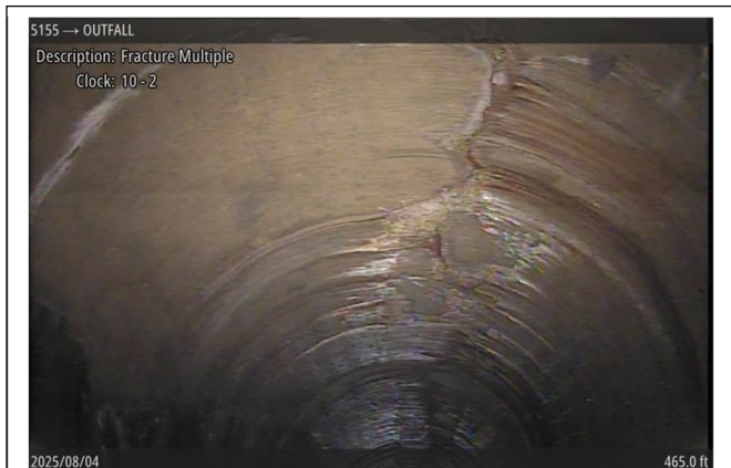
Figure 13 Grade 4 FM in Pipe Segment 5155-OUTFALL
