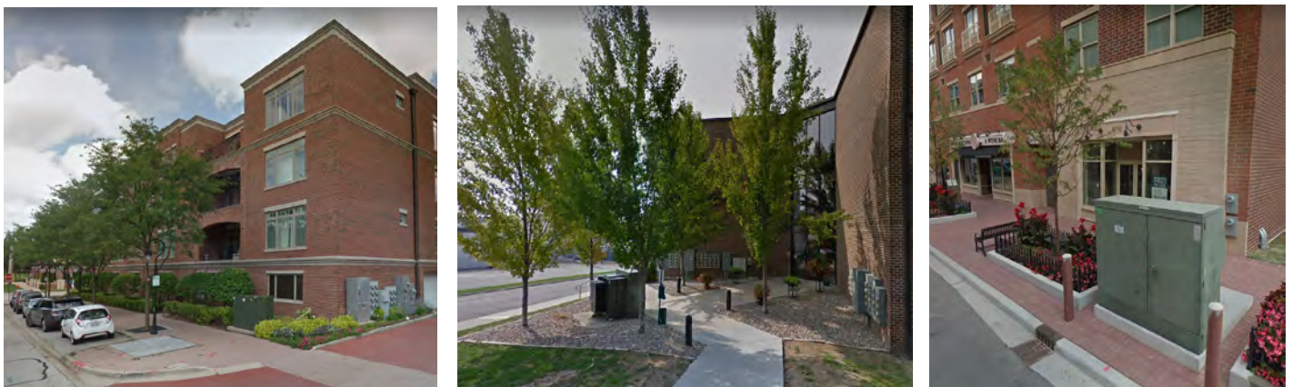
Figure 535-23-20. Examples of Poorly Located Utility Appurtenances on Primary Streets
