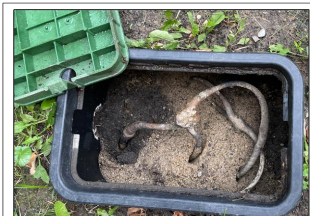
Figure 2 Some Existing Pull Boxes Do Not Require Tools to Access 480-V Wiring
