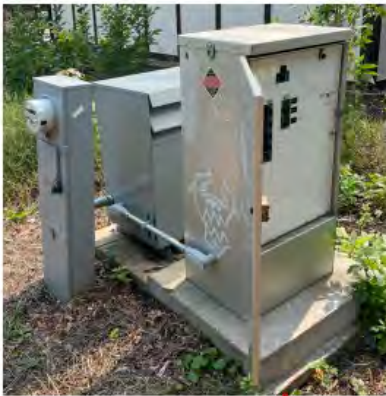
Lighting Control Cabinet
