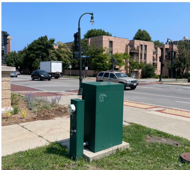
Existing 240V Lighting Panel and Meter
