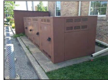
Fire Station Lighting Controller
