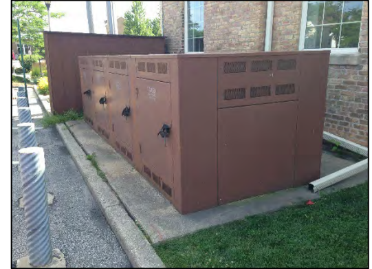
Existing Lighting Control Cabinet
