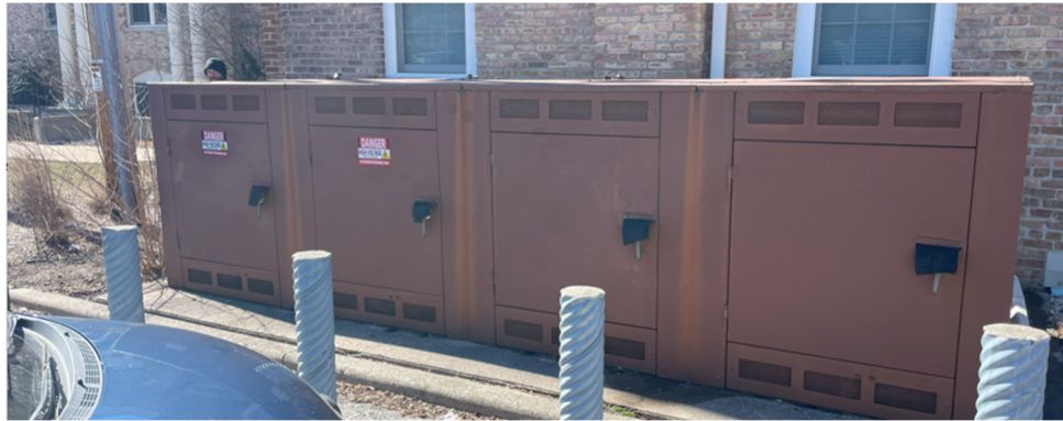
Panel HP4 - Behind North Shore Fire/Rescue Station 83
