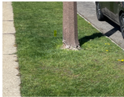
Degraded Light Pole Base
