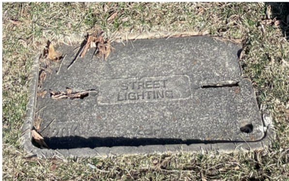
Degraded Handhole for conductor splicing and pulling
