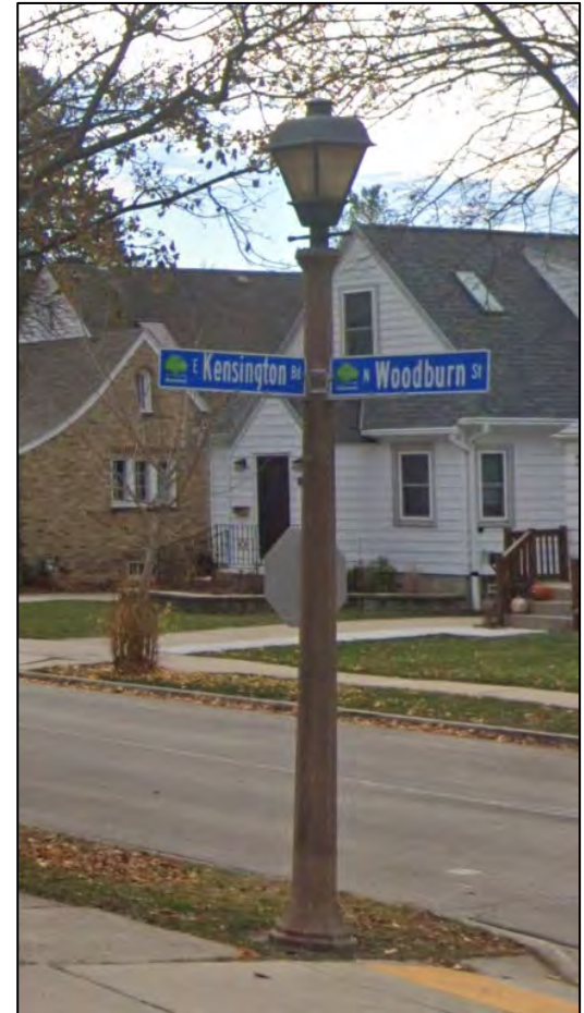
Existing Light Pole with No Handhole to Pull Wires
