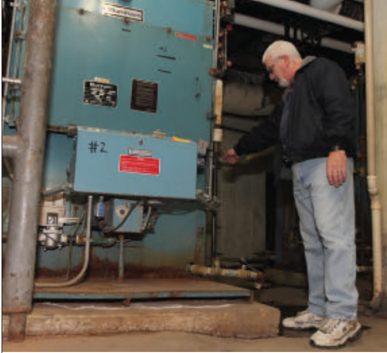
Working Forman Tony Seidita adjusts the controls on a soon-to-be-replaced Burnham boiler at Atwater Elementary School.
